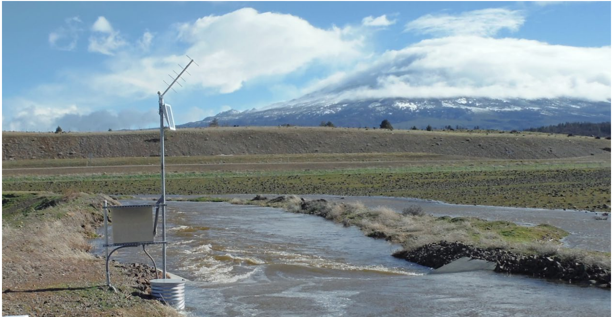
Figure 1 Image of a telemetered stream gage installed by DWR and operated by Montague Water Conservation District on the Parks Creek Diversion Channel in Siskiyou County
