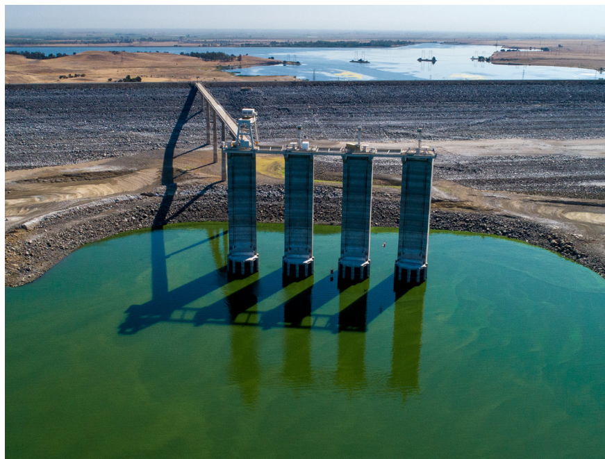
Top: The intake structure at San Luis Dam in August 2021. A danger advisory was issued in September warning people and their pets to avoid physical contact with lake water because of the potential health risks from algal toxins.
