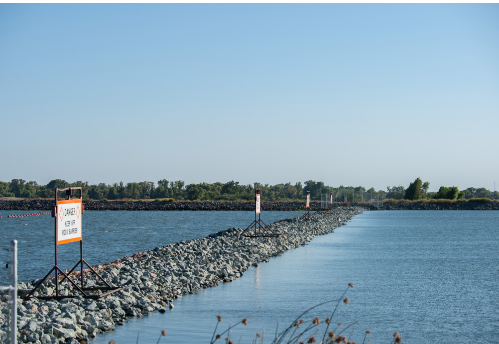
Below: Temporary emergency salinity barrier installed at West False River in the Delta
