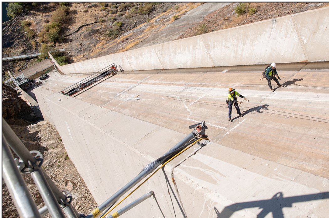
DWR staff assess the gated and emergency spillway for the Pyramid Dam Modernization project in Los Angeles County. Source: Department of Water Resources
