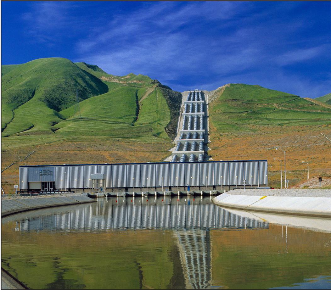
The Ira J. Chrisman Wind Gap Pumping Plant, located just west of Interstate Highway 5 in Kern County. The pumping plant with four discharge lines provides the third in a series of lifts culminating at the A.D. Edmonston Pumping Plant to move the water across the Tehachapi Mountains. Source: Department of Water Resources
