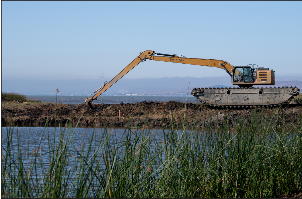
An excavator breaches a levee for the Tule Red Tidal Restoration Project, the first restoration project to break ground in compliance with the U.S. Fish and Wildlife mandate for 8,000 acres of tidal habitat to protect threatened or endangered species. The breach allowed brackish tidewaters to return to more than 400 acres of habitat for Delta smelt, longfin smelt, and Chinook salmon. Source: Department of Water Resources
