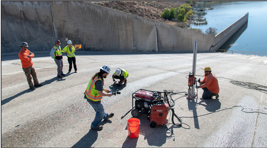
As part of the Castaic Dam Modernization Program, DWR and its contractors take core samples from the Castaic Dam's stream release chute. Castaic Lake State Recreation Area is located in Los Angeles County. Source: Department of Water Resources
