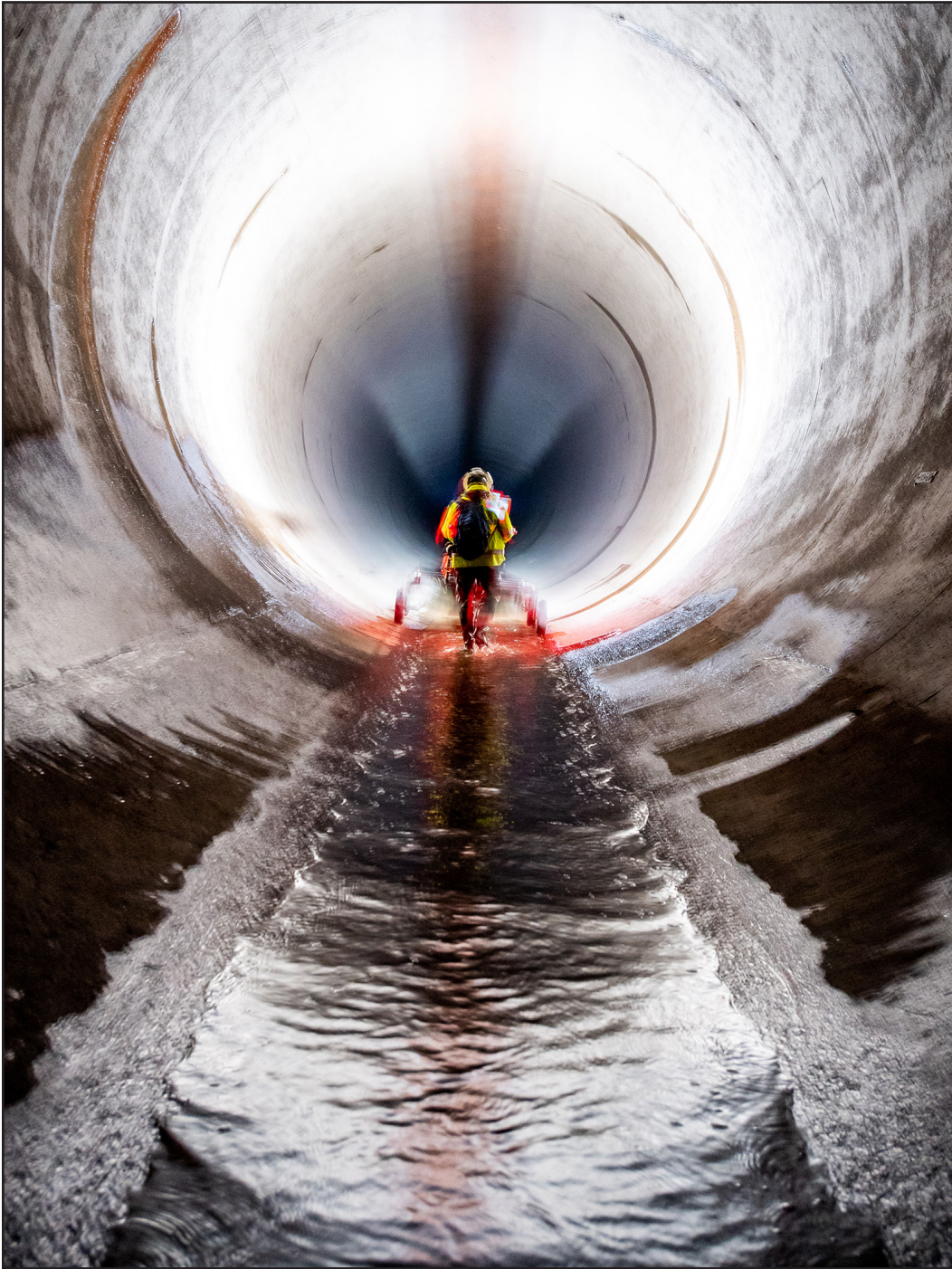
DWR contractors use three-dimensional terrestrial LiDAR (laser scanning) to inspect and survey the Carley V. Porter tunnel, which is 20 feet in diameter and runs more than 25,000 feet across the Tehachapi Mountains in Kern County. Source: Department of Water Resources
